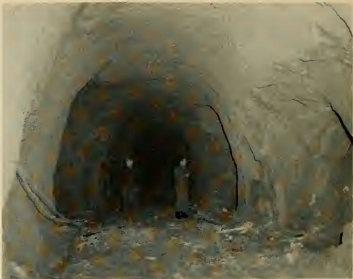
Photo No. 26.—Yoshimatsu plant. Tunnels during construction. Soil is tufa (compacted volcanic dust).
